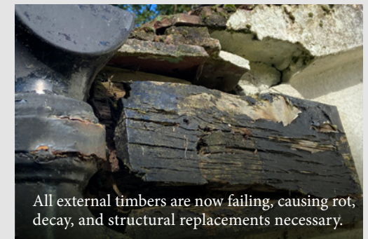
The entire roof structure needs urgent attention. Replacement of framework and tile coverings.
